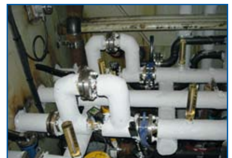
Heetwater- en bunkermanifolds.
